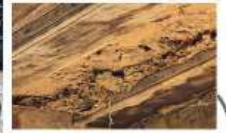
DUE TO THE EXPOSURE TO MOIST CONDITIONS THIS PICTURE TELLS US HOW THE DECAY OF THE TIMBER HAS TAKEN PLACE HIGHLIGHTING THE ROTTEN PART .
