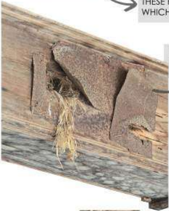
THE LINTELS ARE DAMAGED BY THE PESTS AND OTHER TIMBER INWADERS , MAKING IT A HUGE SURFACE AND BIRD'S NEST IN THE END
