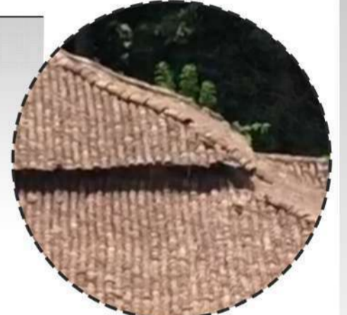
DISPLACED AND BROKEN TILES INDICATE STRUCTURAL MOVEMENT OR WEATHER DAMAGE.
