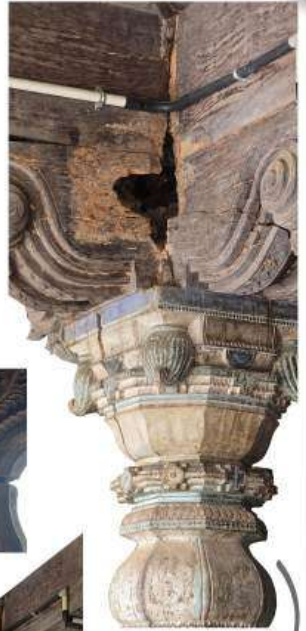
THIS PICTURE AGAIN TELLS US THE DETERIORATION OF THE COLUMNS . EXTENSIVE PEST ATTACK HAS MADE THE CORE OF THE COLUMN VERY WEAK AND IS AT THE EDGE OF COLLAPSING .
