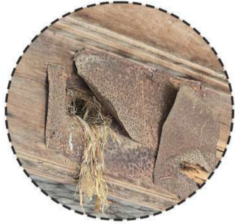
FRAYING AND DAMAGE SUGGEST INSECT ATTACK AND AGING.
