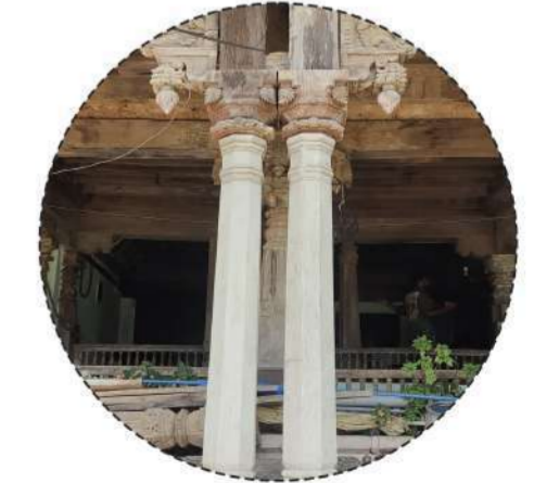
MINOR STAINING AND DAMPNESS AT THE BASE.
