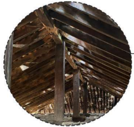
UNEVEN RAFTERS; SIGNS OF SAGGING OR DEFORMATION.
