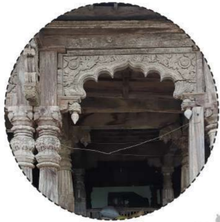
SURFACE DARKENING AND MORTAR LOSS DUE TO WEATHERING.
