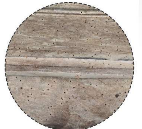
EVIDENT EROSION AND PITTING SUGGEST WEATHERING AND SALT ACTION.
