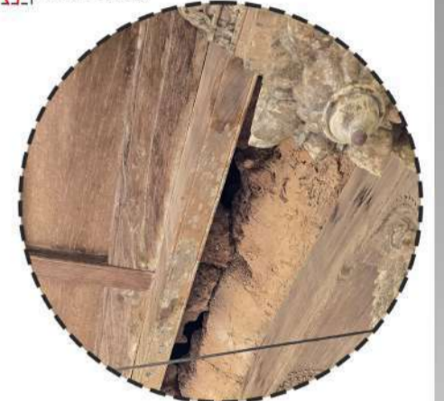
SHOWS DECAY, SPLITTING, AND SIGNS OF INSECT INFESTATION
