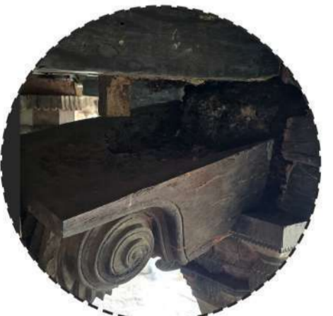
INDICATES STRUCTURAL MOVEMENT OR SETTLING.
