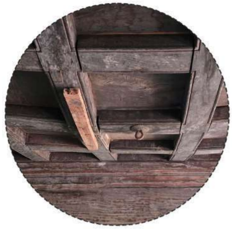
DEFLECTION, INDICATES STRUCTURAL STRESS.
